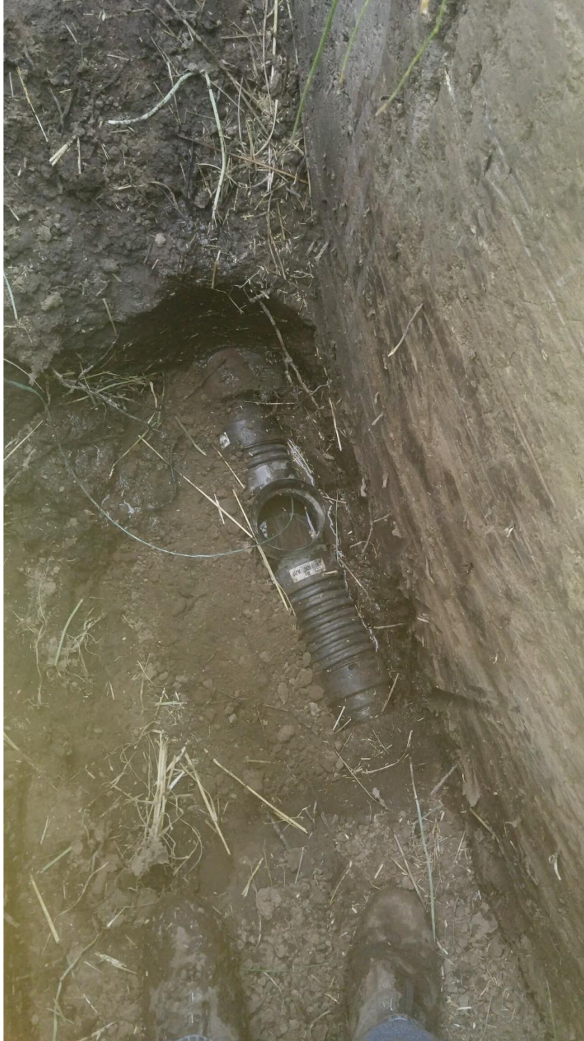
Figure A.3. Photograph of where a backhoe was used to dig down to the artificial drain line while pulling rope to then pull the fiber optic cable.
