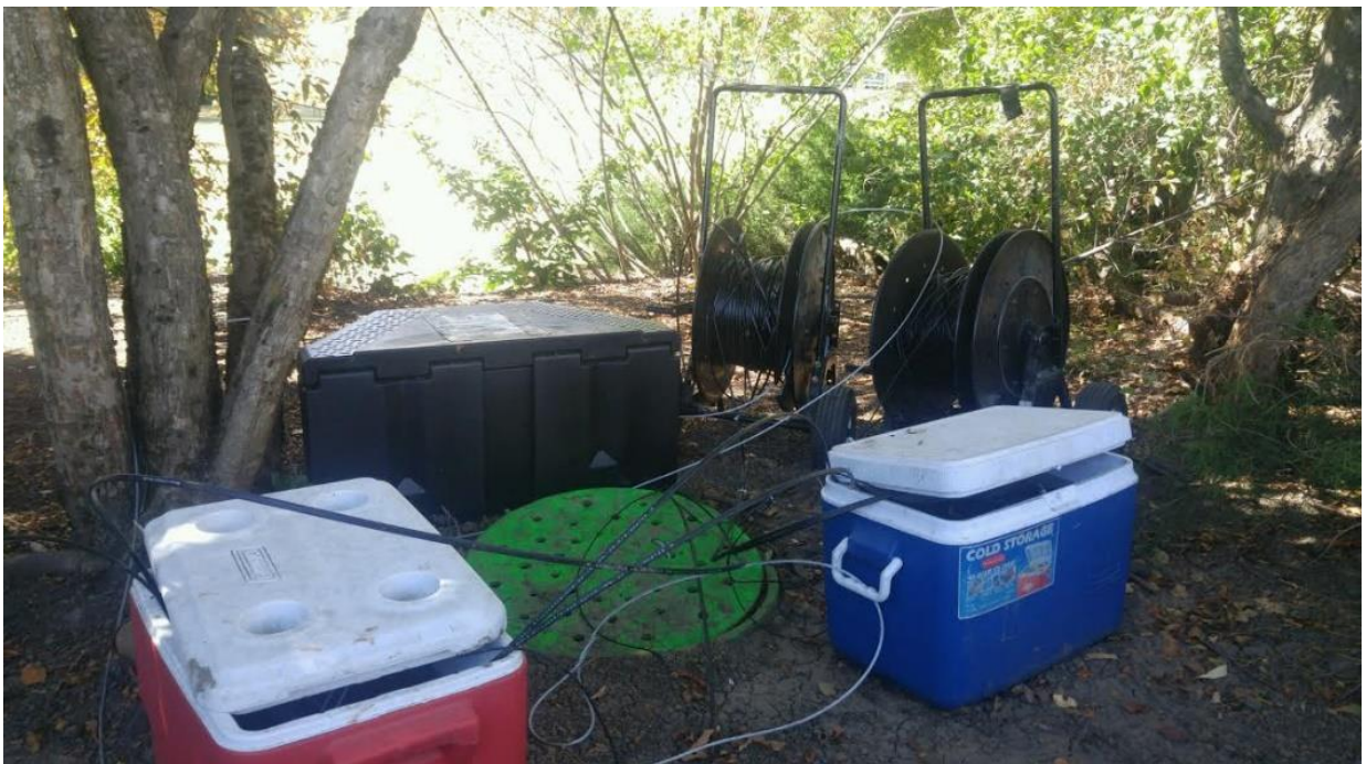
Figure 4.3. Photograph of fiber-optic cables entering the storm drain and the coolers used for calibration baths.
