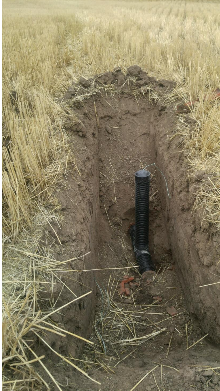
Figure A.4. Photograph of where “T-junctions” were put into the artificial drain lines.
