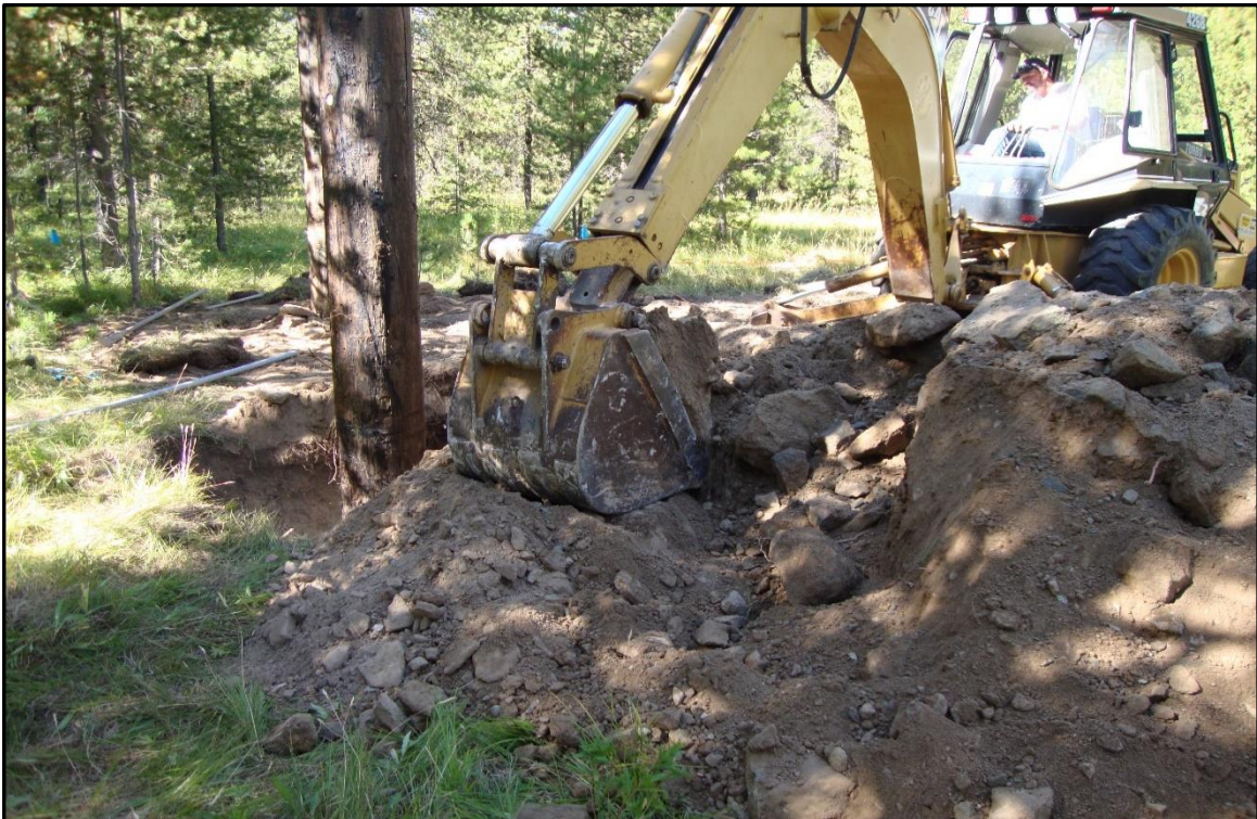
Figure 5-17. Photo taken during the excavation of the holes for the power poles that support the Island Park north site observation tower. Note the presence of large cobbles.
