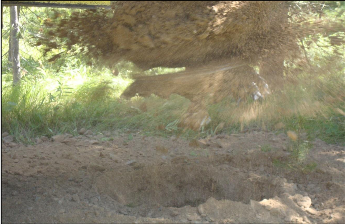
Figure 5-16. Photo taking during the excavation of the holes for the power poles that support the Island Park south site observation tower showing the soil texture. Note the presence of rocks in the soil profile.
