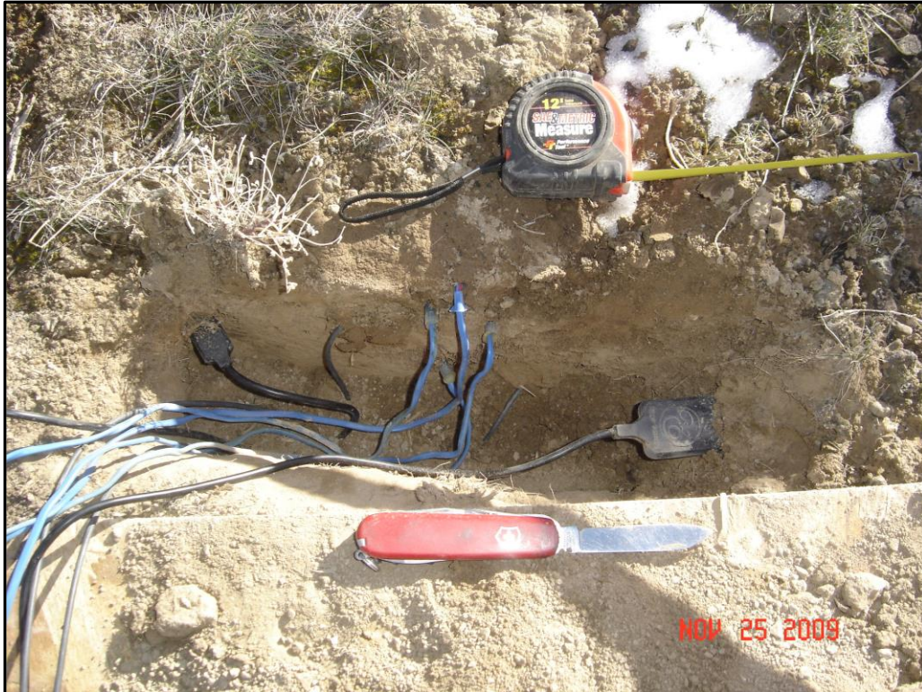
Figure 1-8. View of installation of thermocouples and soil heat flux plates in a soil heat flux subsite. at the Hollister EPSCoR flux site. Installations were similar for the Island Park EPSCoR site. Photo by R.G. Allen
