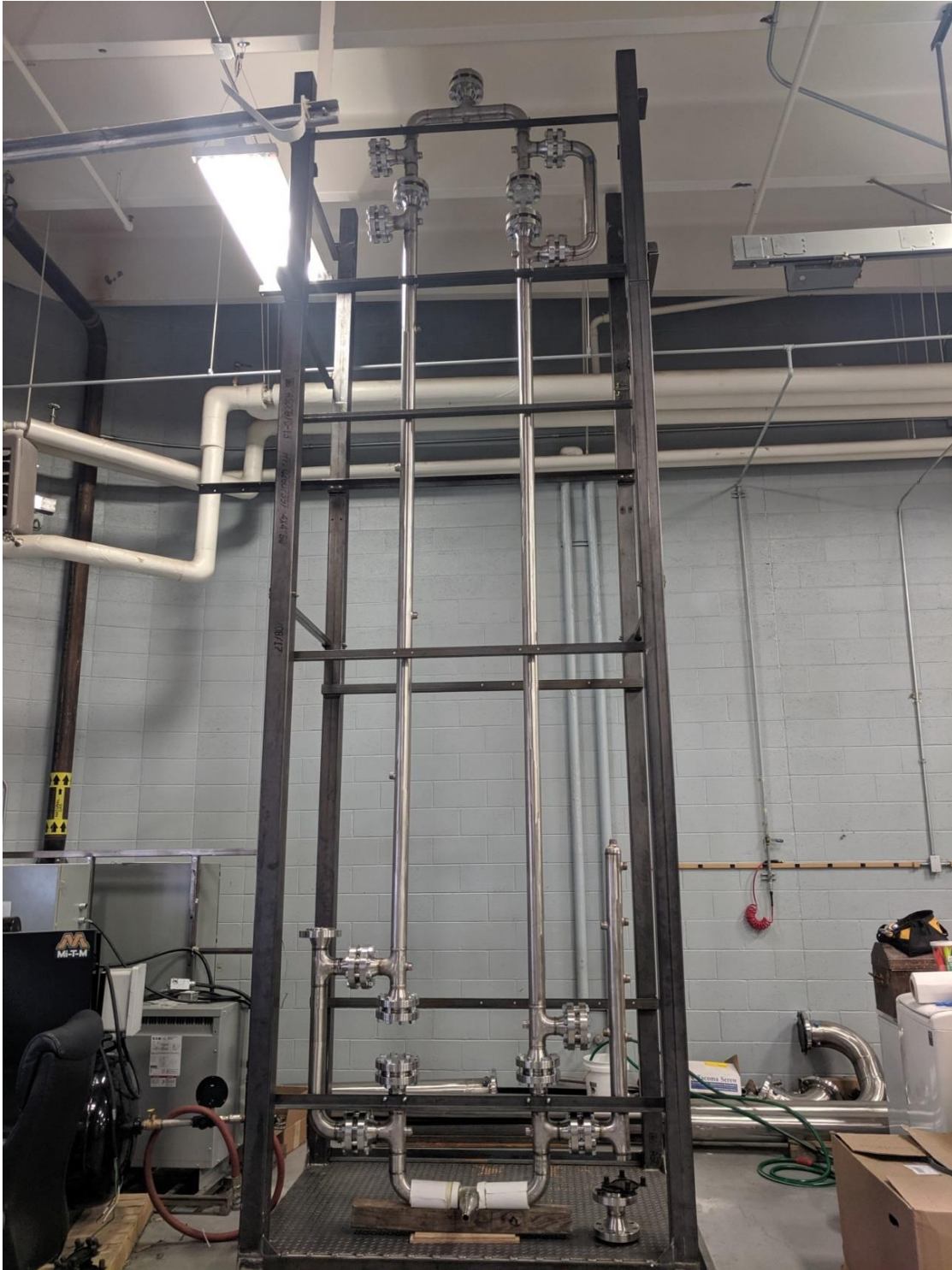
Figure 6-19 – As-Built Test Rig
