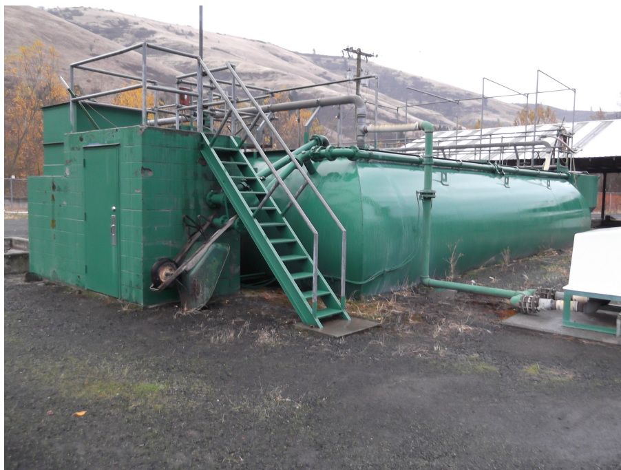
Figure 22. City of Juliaetta centralized wastewater treatment plant, 2017.
