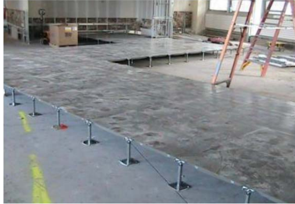
Figure 1.11 UFAD: Under-floor air distribution system construction at Sustainability Base; Poll 2010
