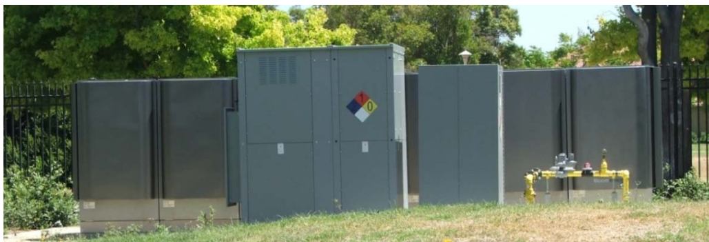
Figure 1.3 Bloom Energy Box: Solid oxide Bloom Energy fuel cell at Sustainability Base converts methane into CO 2 and H 2 O and generates energy in the process; Vanhoozer 2012
