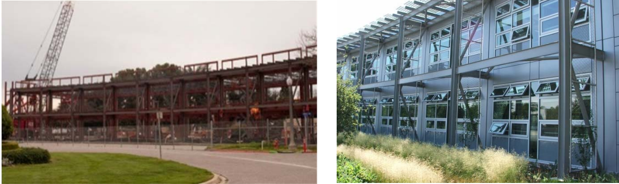
Figure 1.20-1.21 Pre and Post Images: Sustainability Base under construction in August 2010; completed July 2011; Vanhoozer 2010, 2011
