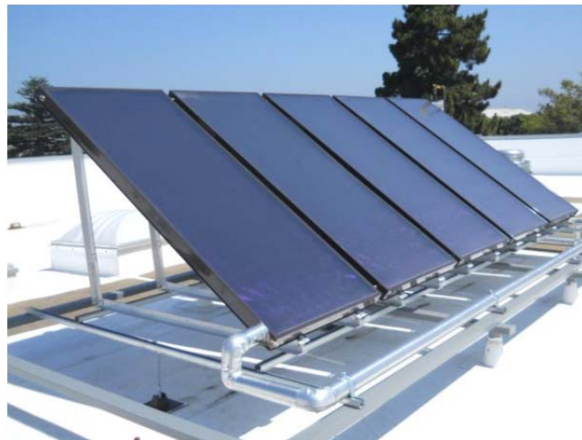
Figure 1.5 Heating Water: Solar collectors are used to heat the water used in sinks and showers in Sustainability Base; Schuler et al. 2010
