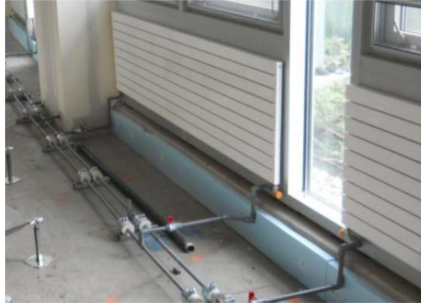
Figure 1.9 Radiant Heat: Wall-mounted radiators heat the building in winter months; Schuler et al. 2010
