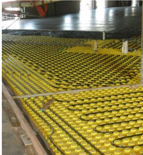
Figure 1.11: An image of the Viega radiant system before concrete is poured at the CSHQA site [25].
