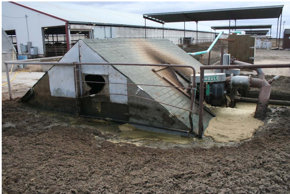
Picture 3. 12 Foaming event and blown window
