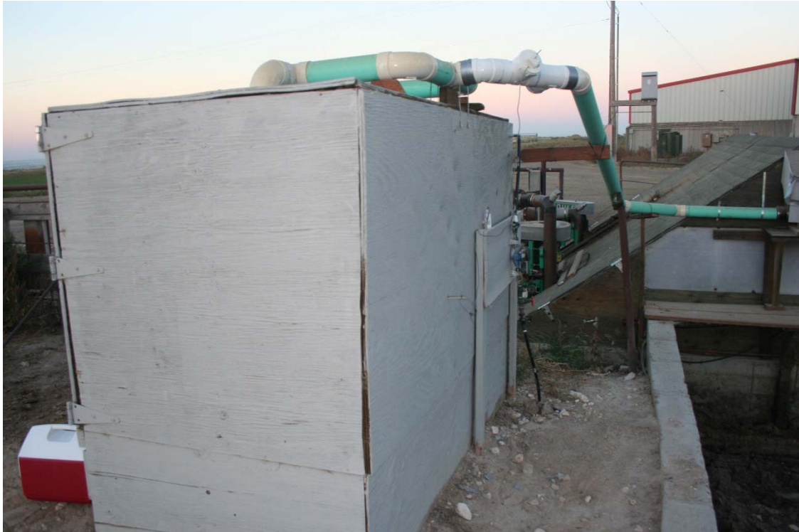
Picture 3. 5 View of pipe from extraction fan to plenum
