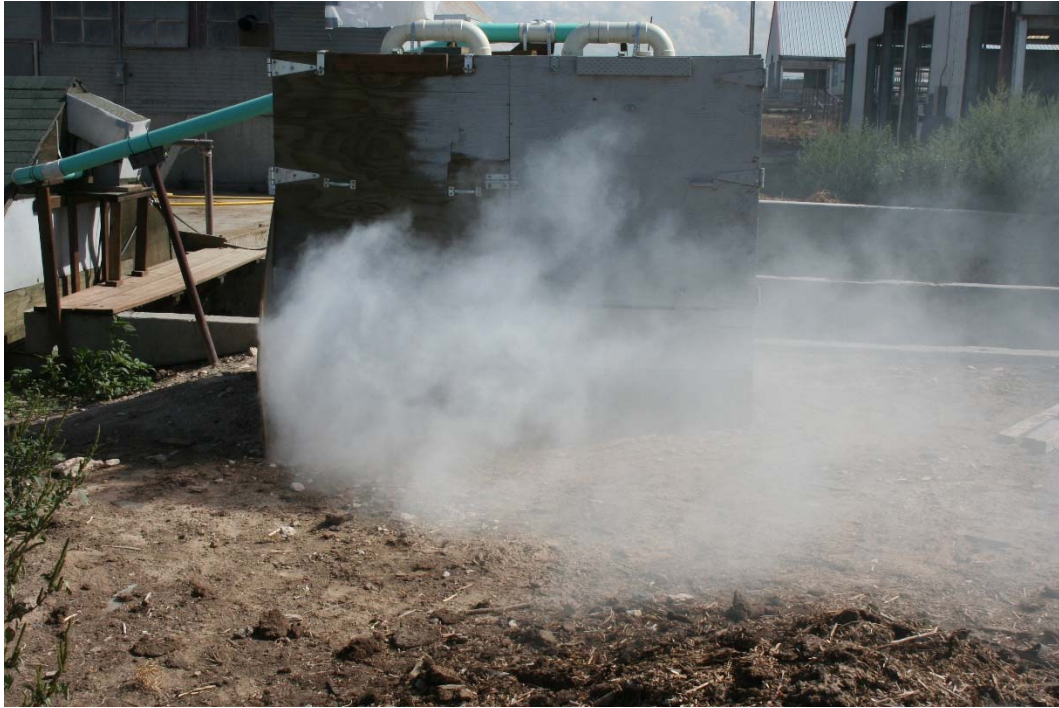
Picture 3. 9 Filter smoke test
