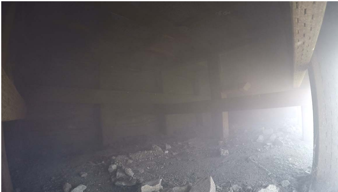
Picture 3. 10 Smoke test filter below filter outlet view
