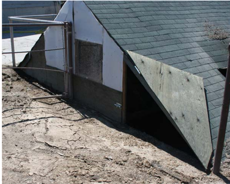
Picture 4. 19 View the “A” side, inspection door, and clear plastic coverage
