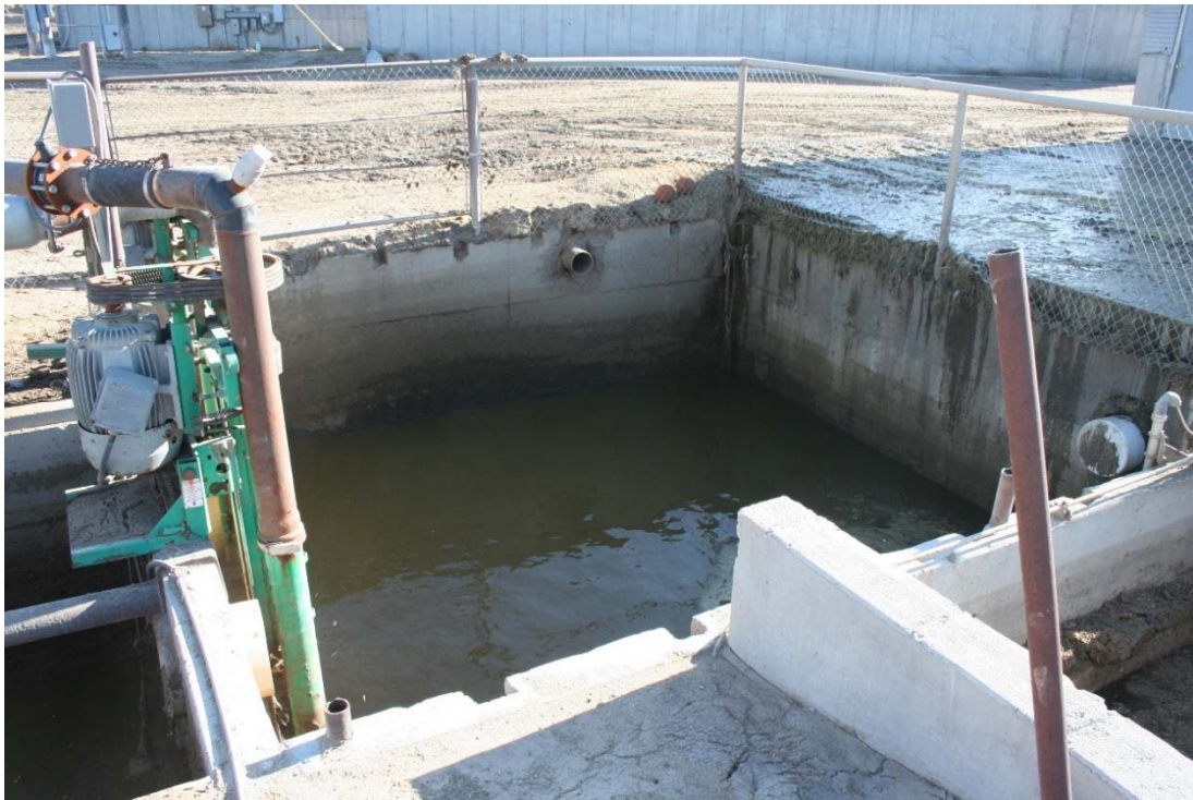
Picture 3. 1 Dairy manure collection pit before any work on the project started
