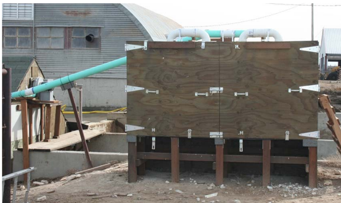
Picture 4. 6 Front view of filter and plenum
