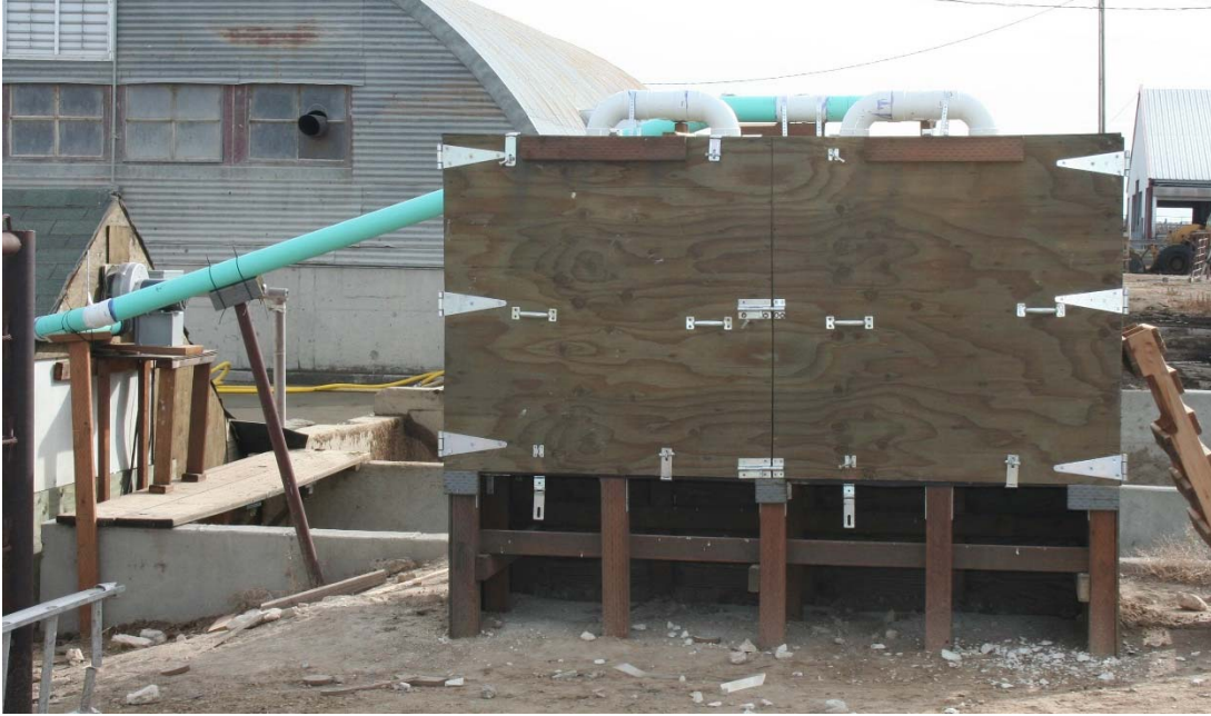
Picture 3. 7 Front view of filter with connecting pipe and plenum
