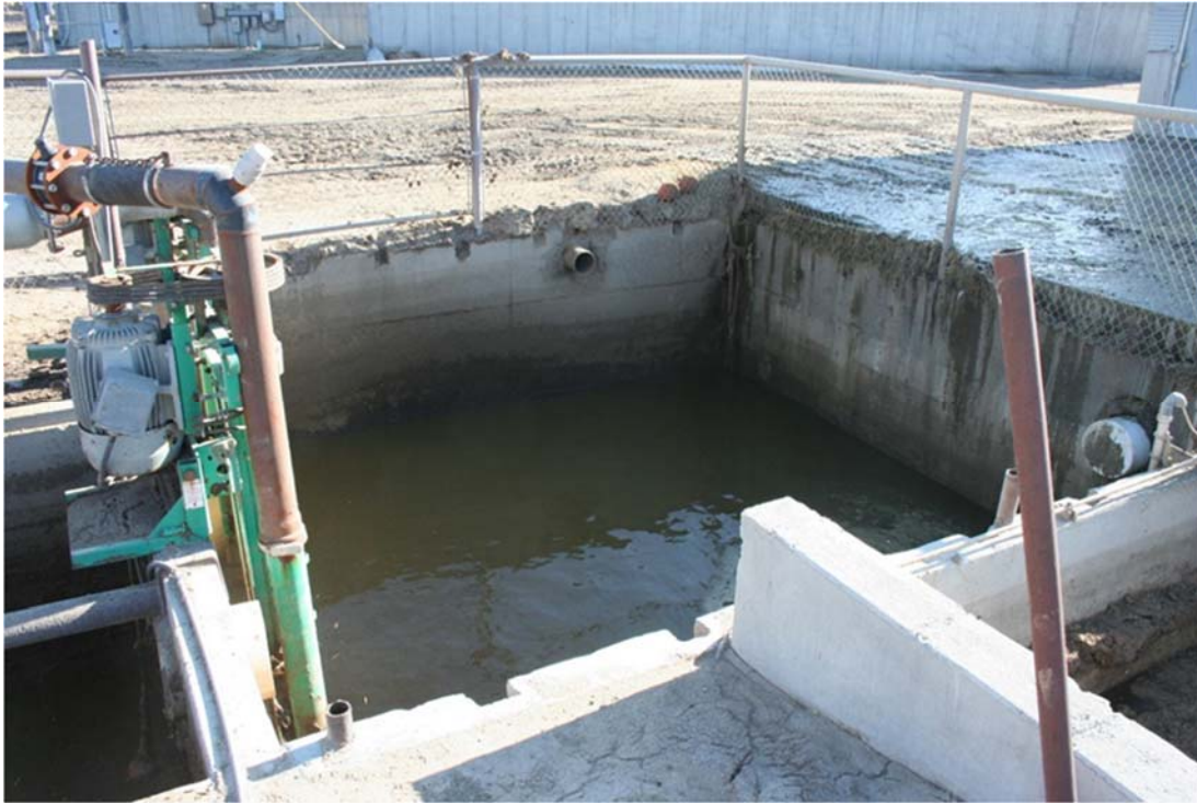
Picture 4. 15 Dairy manure collection pit before any work on the project started
