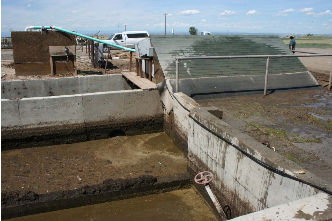
Picture 3. 3 Roof like pit cover connected to the zeolite filter
