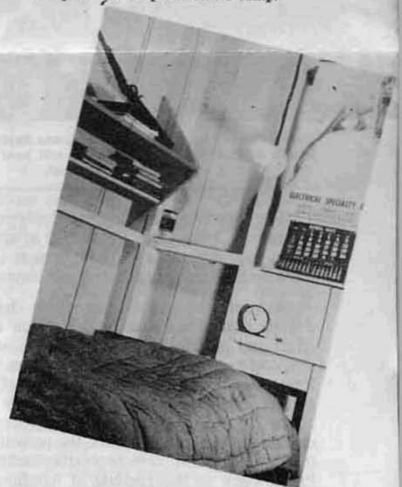
Above, a light over every bunk with a plug-in, convenience outlet, in base of lamp to permit use of radio, electric razor, extra light or other electrical gadget.
