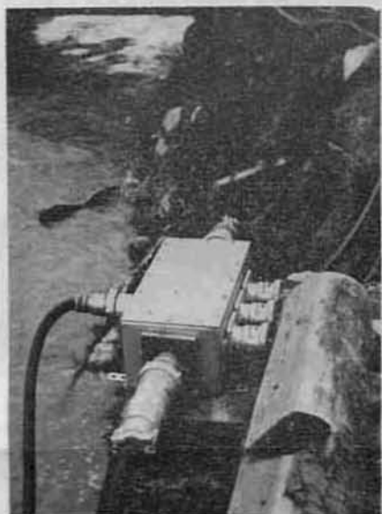
Above, distribution box at Camp 58. Note three outlets for single phase power and the outlet at opposite side of box for three phase power. The same connector is used here as elsewhere about the system and provides complete protection of the socket. Main line cable is laid along stream bank—it needs no protection from weather—neoprene jacket guarantees long life.
