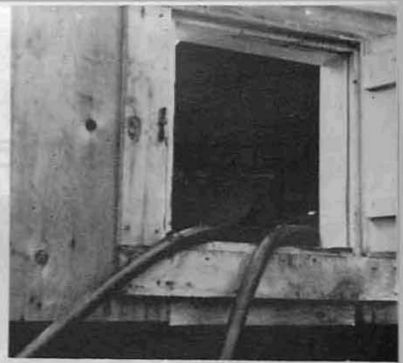
Above, the main line cable, 1 3/4 inch diameter, neoprene jacketed to resist sunlight and oil, leaves the power house through a small trap door to loop the entire camp.
