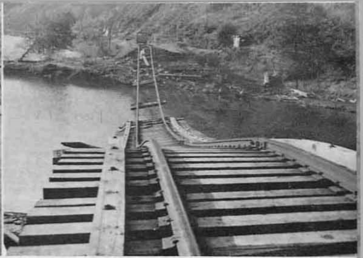
aged and fill was taken out by force of water (pictured above).
