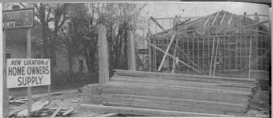
Above, new yard of Home Owners Supply taking shape. Manager Wayne Anderson cheerfully admits it to be the best laid out yard in the northwest. At right . . . rear view of yard showing ample storage space which will permit good customer service.
