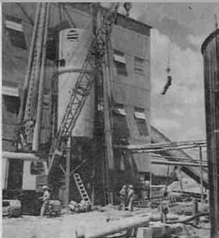
Construction worker going aloft to work on addition to Clearwater pulp and paper mill powerhouse and recovery room.
