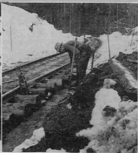
Above—Sections of track had to be dug out, raised and shimmed up with wood slabs, then ditched to drain away the water from rotting snows.
