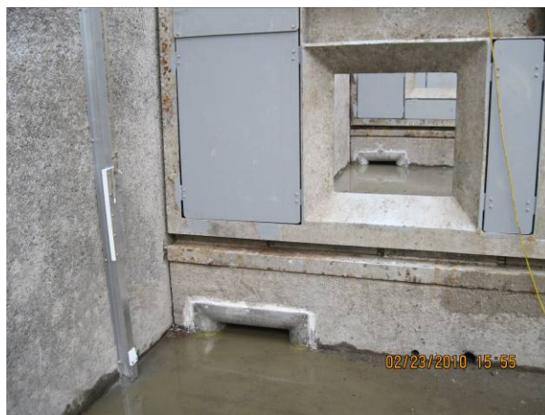
Figure 1. Photograph depicting openings cut into the bases of adjustable-overflow weirs in the Oregon-shore fishway at McNary Dam, 2010.
