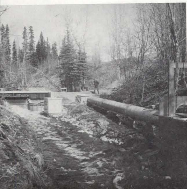
Fig. 13. Upstream view of the 18.3 m culvert facility showing the position of the headbox, tailbox and dam (1973).
