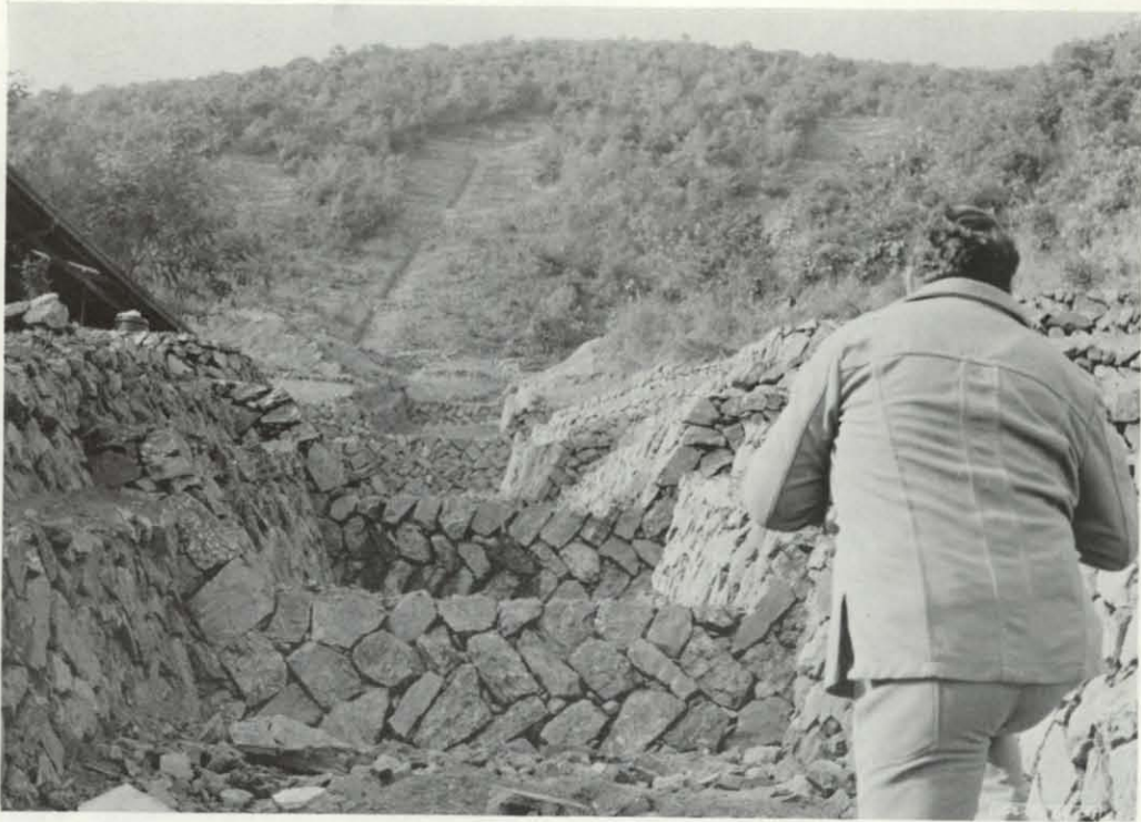
Figure 4. A stone-lined drainage channel has been installed in this slide area. Note walled steps, which reduce the effective channel gradient.
