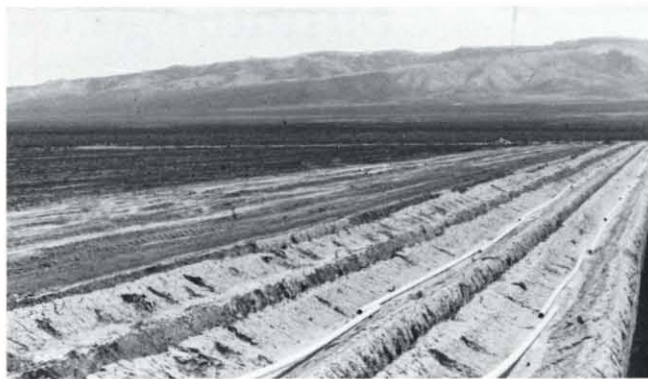
Pipelines are laid out for use in a soil heating project utilizing thermal water in tree biomass production.
