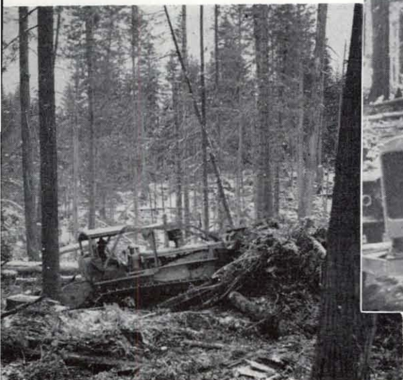
Figure 37. . . . the bulldozer has taken over 30 per cent of the . . . slash piling job.
