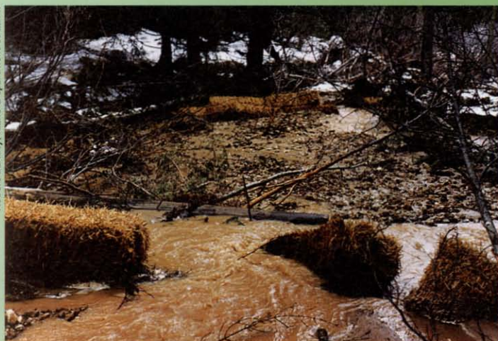
Failed staw bale check dam.
