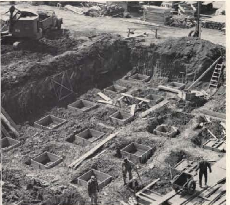
Such work as pouring molds for supporting columns fascinated the passersby throughout the year. The Classroom building will be finished in January, 1951.
