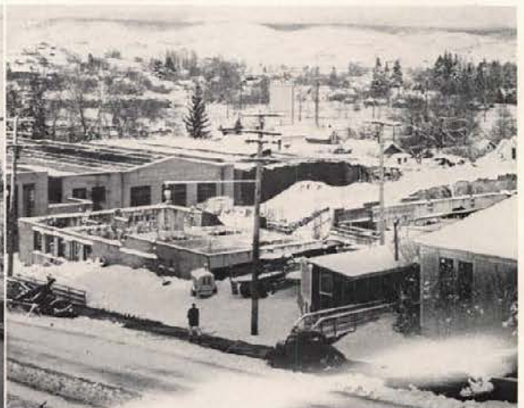
The work on the Engineering Classroom Building, which was well started last fall, slowed to a standstill with the deluge of mid-winter snow. The foundations are seen above, with the Kirtley addition lying beyond.
