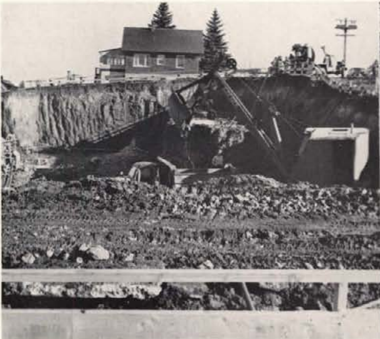
Initial excavation for the Engineering Classroom building tore up the land across the street from the Navy building.
