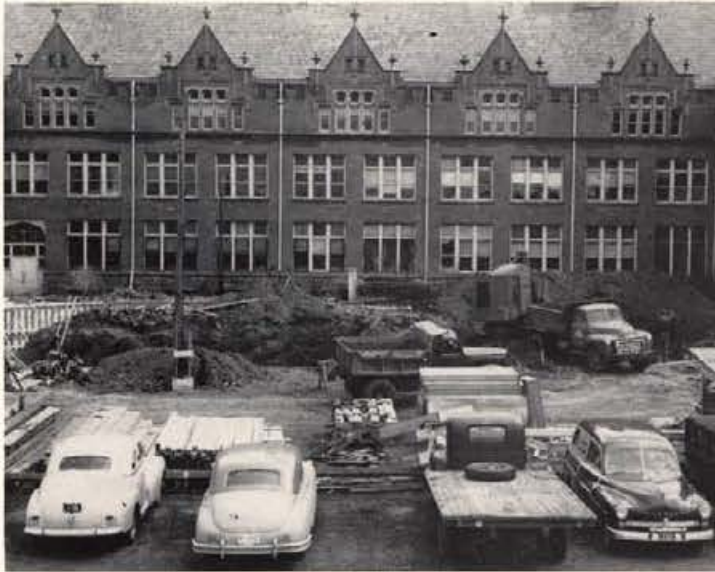
With the wings of the Administration Building on either side, the new Administration Building annex, foundation work of which is shown above, will house the Registrar, Bursar, and other administrative offices of the University.
