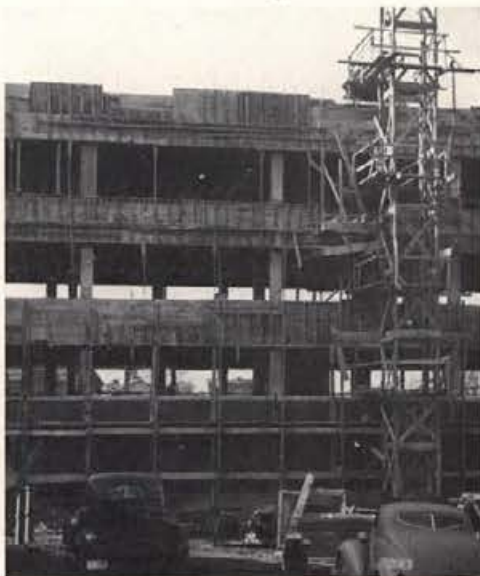
The Agricultural Science Building, standing like a gaunt skeleton silhouetted against the sky, was rushed to external completion before the winter snows set in.
