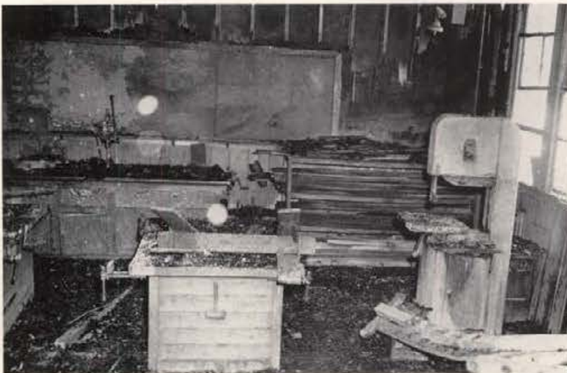
AN EARLY MORNING FIRE on March 20 razed the interior of the northwest wing of the Industrial Arts building, causing an estimated $20,000 damage. The building contained power equipment used by the industrial arts classes.
