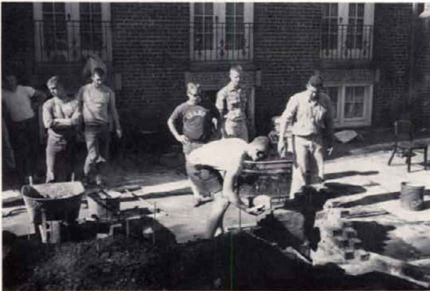
The various living groups are always busy on work projects to help add to the beauty of our campus and here the ATO's install a new sidewalk leading from their driveway to their front door.
