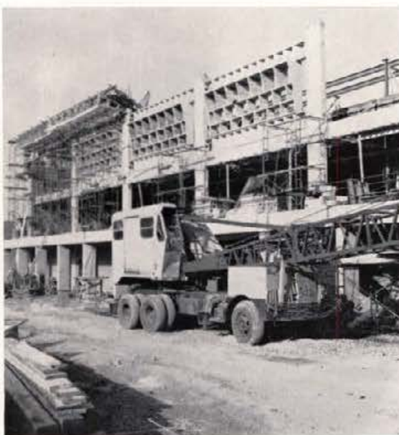
As construction on the new University Classroom Building progresses, one sees that life on this campus includes more than the functions of an active student body.
