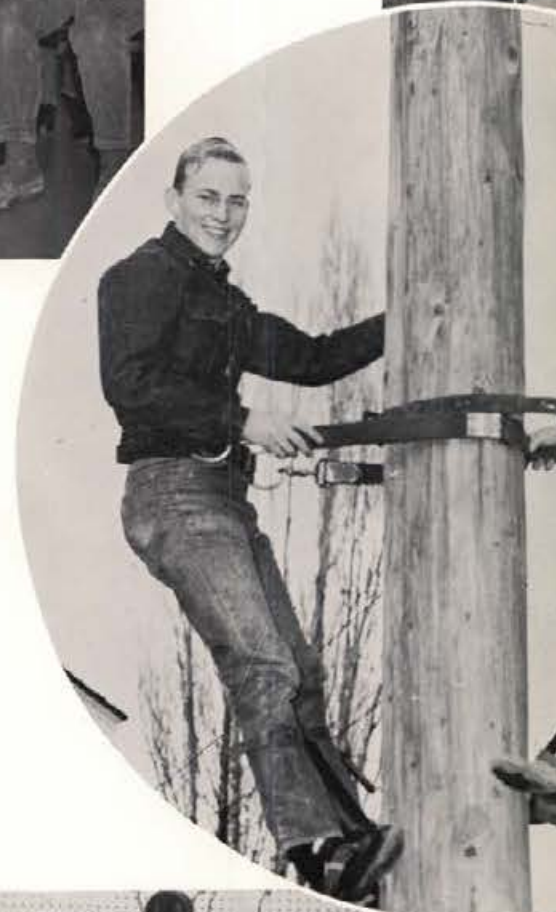
Andy Johnson and Greg Melton, members of the KUOI staff, are busy stringing a distribution system high above the ground.
