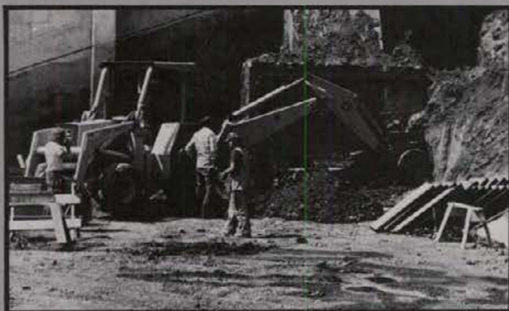
SCOOPING OUT the foundation construction men begin work on the East End Addition.
