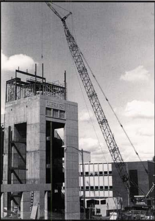
Cranes lowered the steel beams for the library tower into place during the first several months of school.
