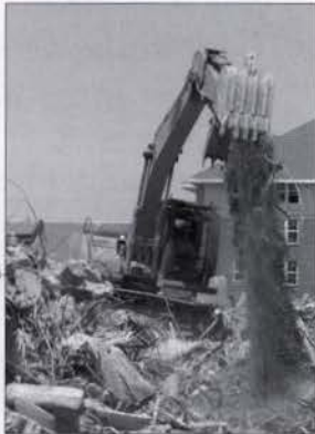
BRIAN PASSEY / ARGONAUT A demolition crew tears down Gault Hall on Monday afternoon in preparation for phase two of the Living Learning Community project.
