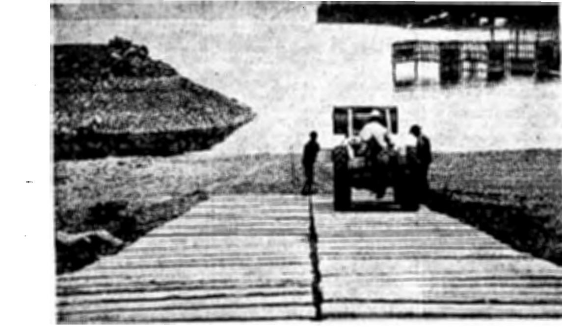
TO HELP IMPROVE public access to Lake Pend Oreille, Idaho Fish and Game Department field men lengthen a concrete boat ramp at Garfield Bay. This is a popular camping area which provides angling for largemouth bass, Dolly Varden, cutthroat, kokanee, and trophy size Kamloops.
