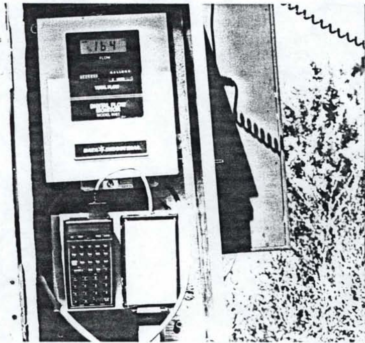
Figure 2. Pumping Station Monitor
