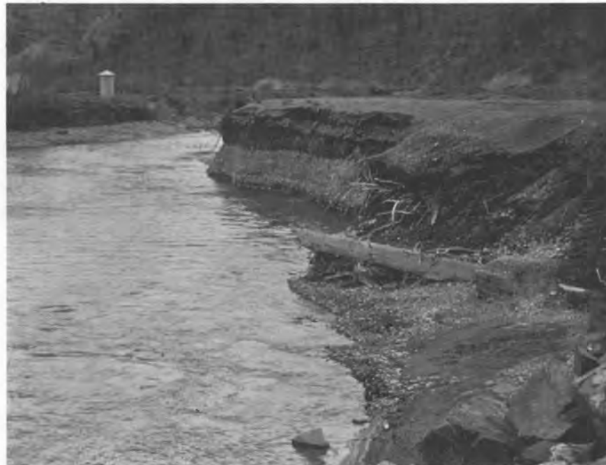
This photo is an example showing the type of stream channel falling under Classification No. 2 Guidelines.
