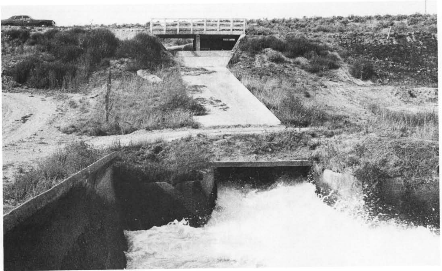
Figure 84. Electric Drop site on the Boise Project.
