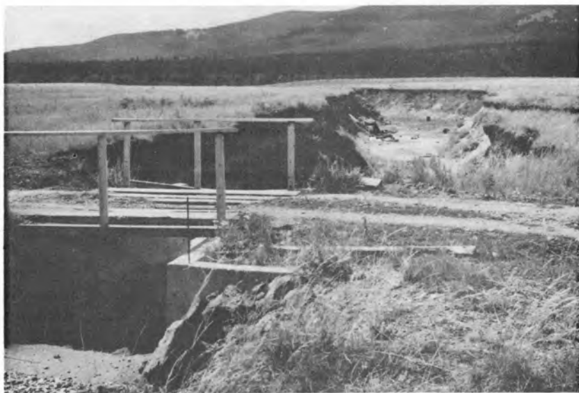
Figure 24. Downstream view of streambed shown in Figure 23 showing serious erosion problems. Eroded material is deposited in an alluvial fan where the stream joins Henry's Lake Outlet.
