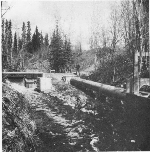
Figure 11. Upstream view of the 18.3 m culvert facility showing the position of the headbox, tailbox and dam (1973)
