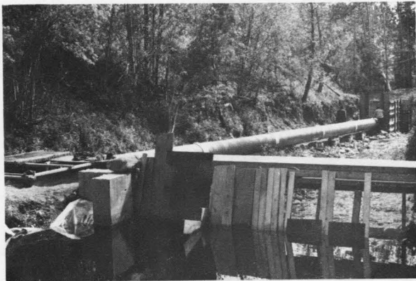
Figure 12. Downstream view of the 30.5 m culvert facility showing the position of the headbox, tailbox, and dam (1974)
