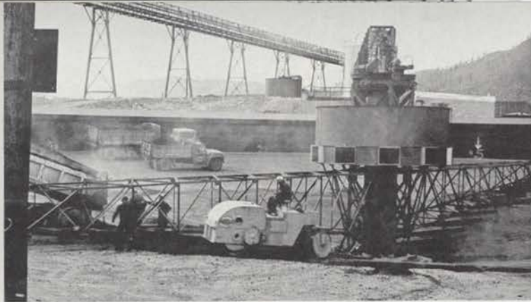
Construction of a new Central Treatment Plant by Bunker Hill Company will settle out dissolved metals in solution by combining them with a lime slurry. This will minimize the amount of toxic wastes into the South Fork and hopefully meet state and federal requirements.
