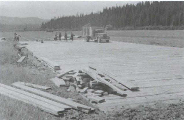
Constructing a landing field in pasture two miles north of Laird Park.
