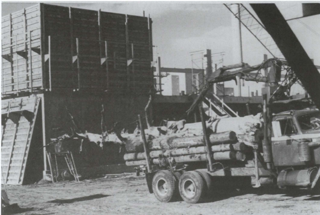
It was nothing short of a miracle that the snag made it intact to the site of the Forestry Building seen under construction in the background. A crane then lifted the old tree over the walls and lowered it to its new home in the west foyer of the building. Courtesy of UI College of Natural Resources.
