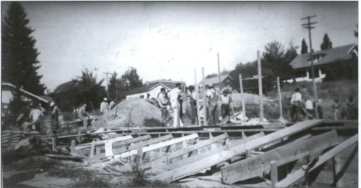
After tearing down Rosenstein's old store, Esser Construction built the Genesee Medical Building in 1948. Wendy Woods Collection, courtesy of Earl Bennett
