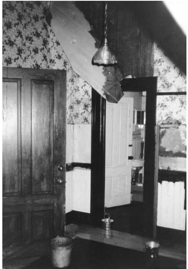
A broken radiator pipe in the attic resulted in water damage on lower floors, mostly in the kitchen area and unrestored rooms. (1993)
