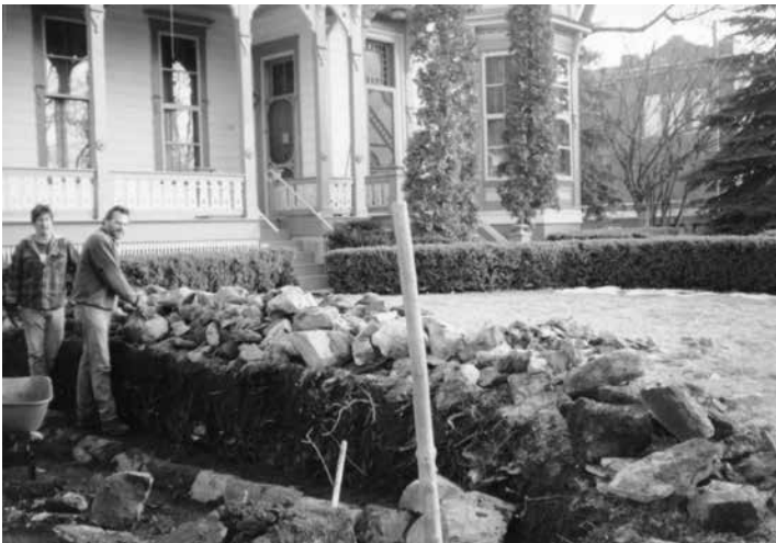
Workers from North Country Landscaping rebuild the rock wall at McConnell Mansion. (1999)
