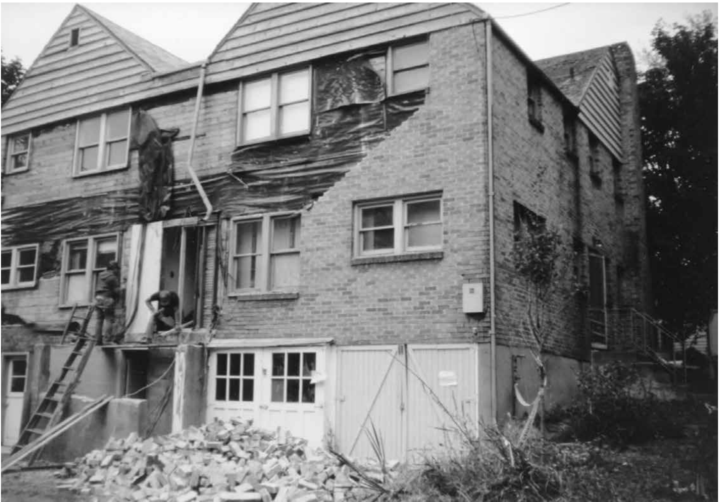
Workers rebuild the south wall of Centennial Annex after removing the stair tower. (1993)
