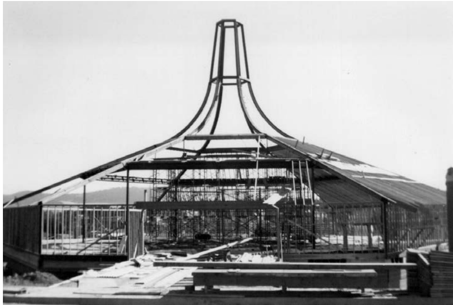
Framework of the roof and spire shows what the final church structure will be.
