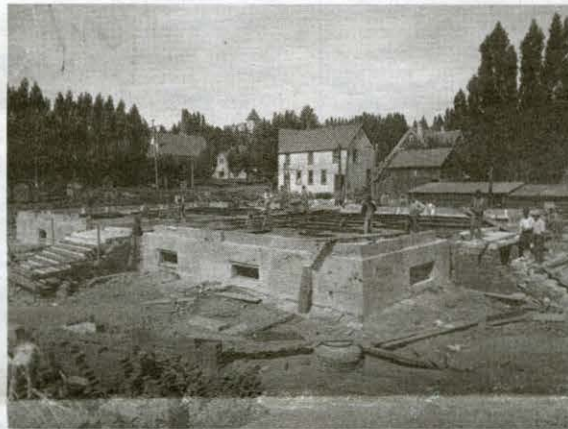
Foundation work for the new Moscow Post Office and Federal Building kicked off in 1909
