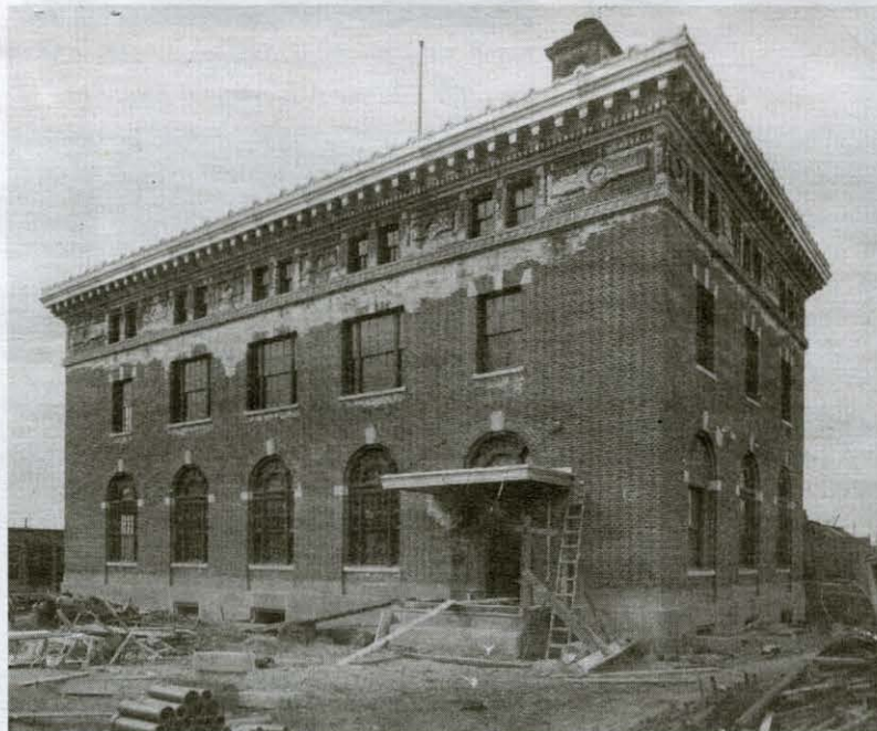
The building as it nears completion in 1911. Both photos courtesy of Latah County Historical Society
