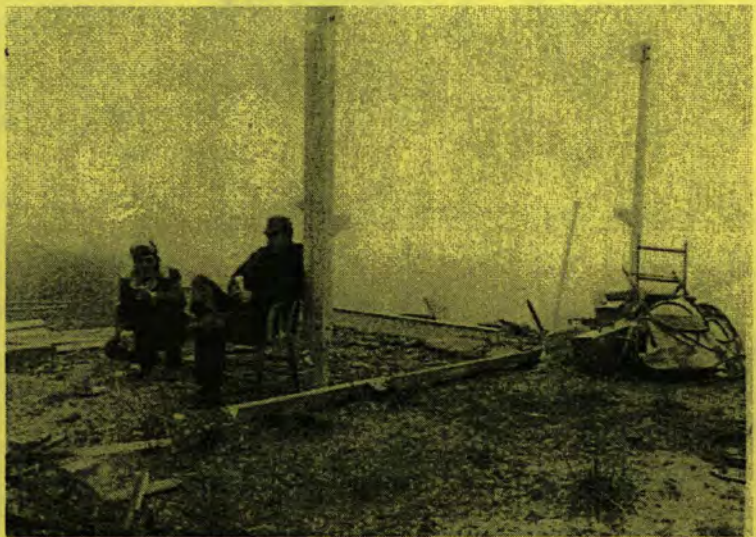
Jim Bulter (left ) and Gordon Fouche taking a break on Lookout Mountain while taking apart the 1957 metal cab to move it to Sheepeater Mountain.
