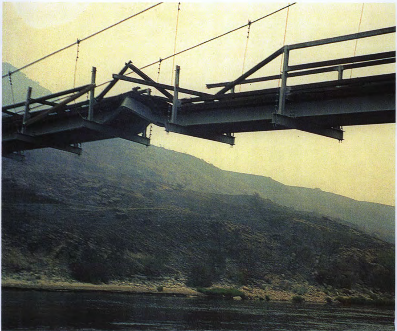
Hot wind lifted the suspension bridge and buckled the foot-wide beam supports.
