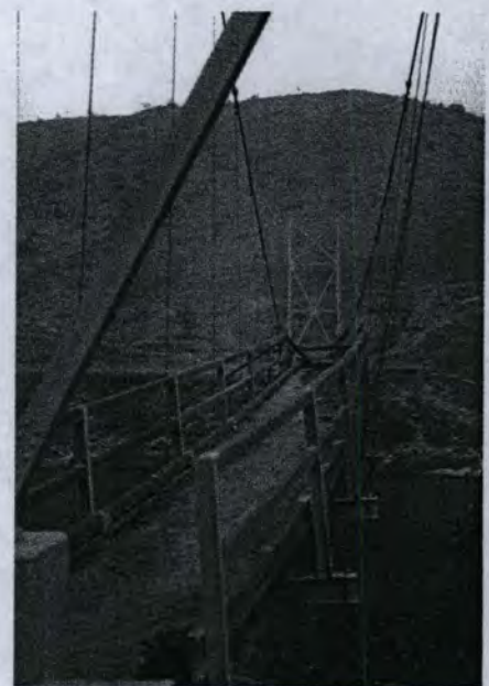
The power of the firestorm twisted this suspension bridge over the Middle Fork of the Salmon River.
