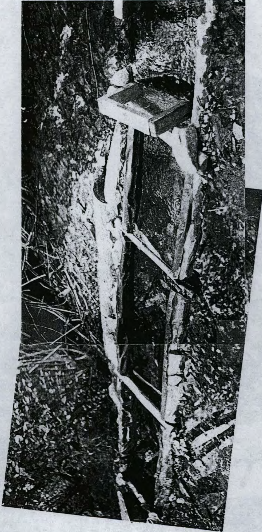
POTABLE WATER SYSTEM WITHIN PIONEER CREEK
