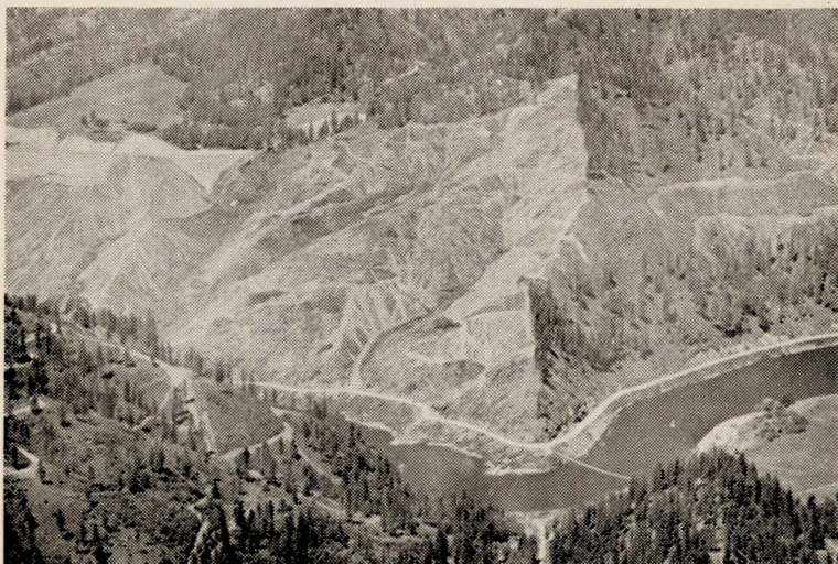
DWORSHAK DAM CLEARING —Early stages of construction at the Dworshak Dam site in 1964 included the clearing work. Above can be seen the first clearing project. Many miles of up-stream forested hill sides remain and it will take several years for completion. The Association has entered into a contract with the Army Engineers to assist them in some of the work and with fire regulations.
