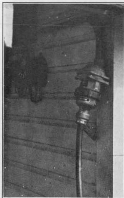
The exposed power outlets are provided in weather-proof fittings
