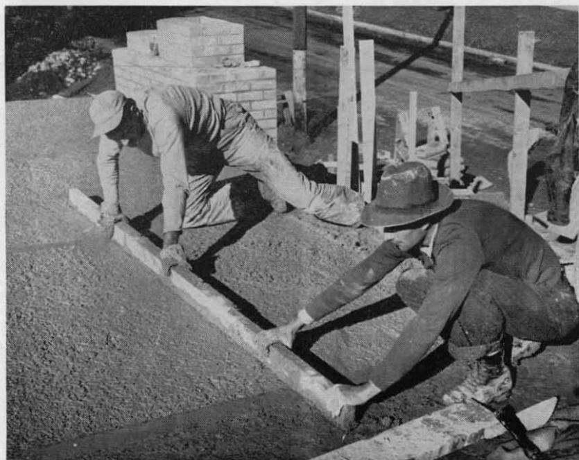
Figure 4.—Roof slab of wood-waste concrete. The screeding operation shown above was followed by smoothing with a steel trowel in 3 hours. Built-up roofing was then applied directly to slab.
