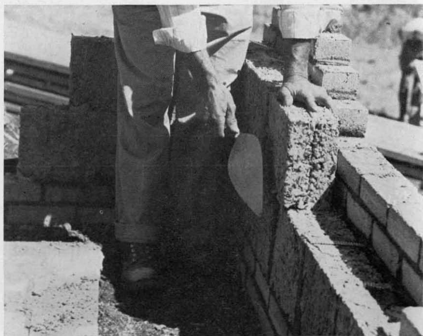
Figure 3.—Insulating block of wood-waste concrete being laid in wall. Outside wall is brick veneer; inside finish may be plaster applied directly to block.
