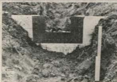
Looking downstream on installed weir. Note the end and bottom contractions and staff gauge location
