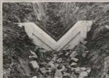
Looking upstream on installed 90°-V notch weir. Note the gravel and rock protecting apron.
