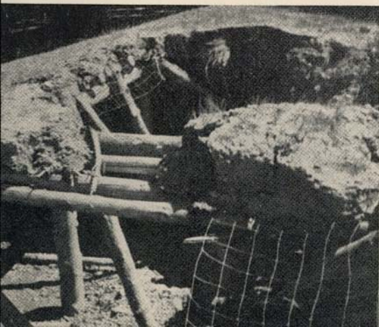
Figure 9.—This is what happens when untreated wood is placed in a cellar. Timber replacements started during the sixth year in this cellar near Thornton. It failed completely the tenth year. Treatment would have assured much longer use.
