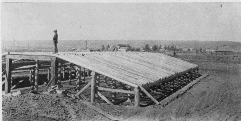
Figure 6—Dugout timbers in place ready for wire and straw. Note heavy rafters laid close together.
