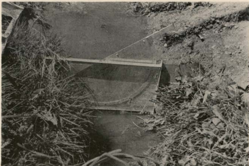
Figure 9. — Rotary control gate used to control the water level in the head ditch.
